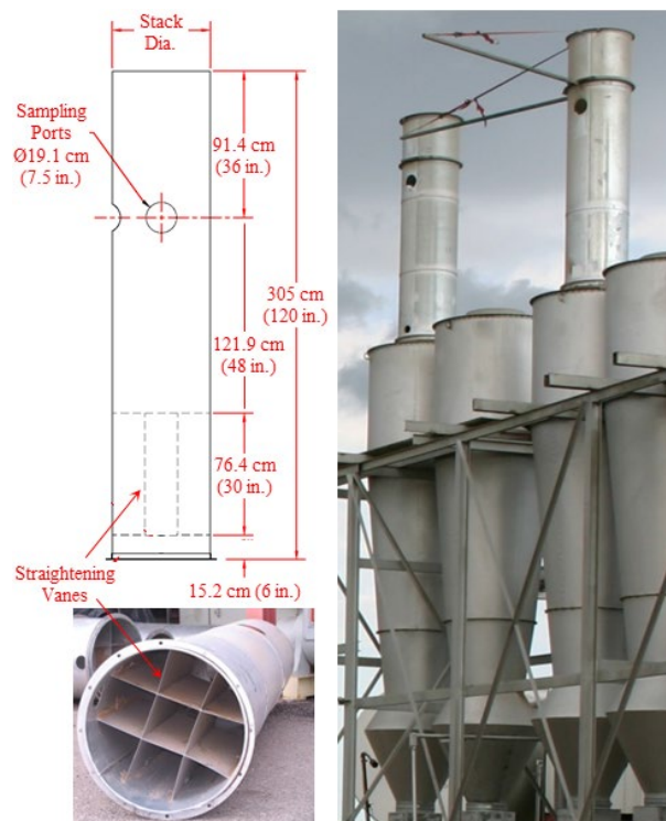
Figure 7. Schematic and photographs of stack extensions with sampling port and straightening vanes (rail attached to extension above sampling port, at right, supports sampling probe during testing traverse).
