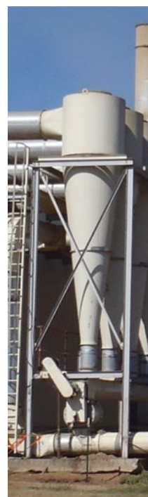
Figure 11. Cyclone design for the tested systems: 1D3D cyclone with 2D2D inlet and standard cone.
