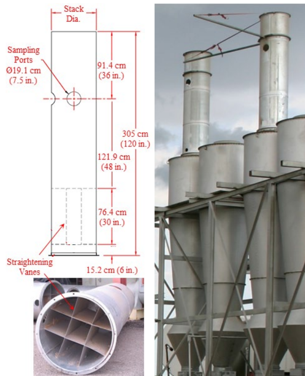
Figure 7. Schematic and photographs of stack extensions with sampling port and straightening vanes (rail attached to extension above sampling port, at right, supports sampling probe during testing traverse).
