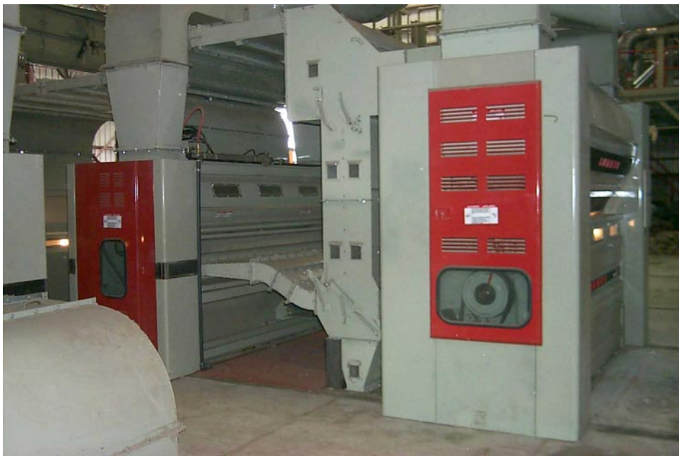
Figure 3. Sentinel™ Lint Cleaner (left) and Model 108 Lint Cleaner (right) installation at Jones County Cotton Gin.
