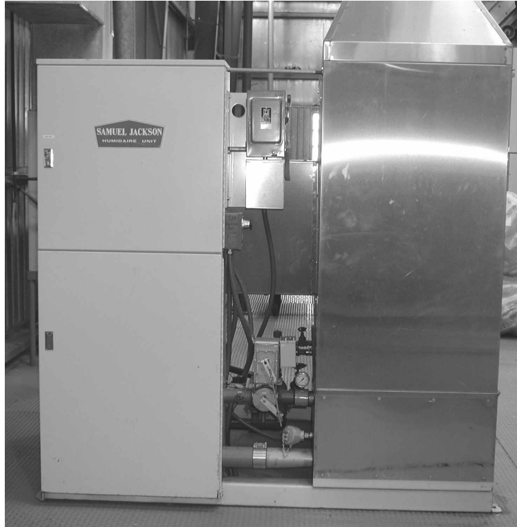
Figure 3. Humidaire Unit used in the moisture restoration system.
