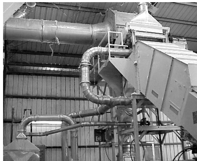
Figure 1. Moisture restoration system at McClendon, Mann, and Felton Gin.
