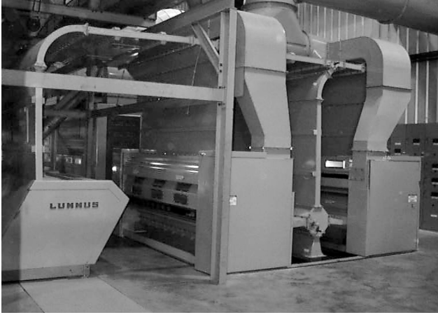
Figure 10. Installation of third Phase II Sentinel™ Lint Cleaner at Sowega Cotton Gin.
