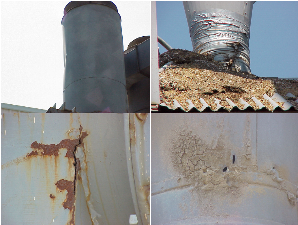
Figure 11. Examples of poor cyclone maintenance (clockwise from top left: dents, joint leaks, wear holes, and stress cracks).
