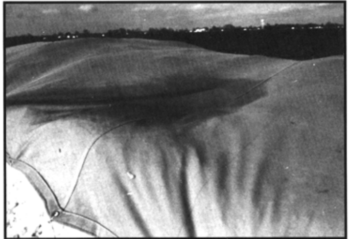
Figure 5. Make modules so that depressions (where water can accumulate) do not exist.
